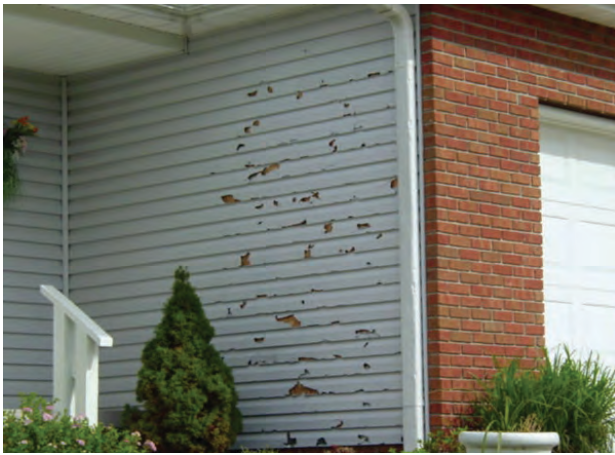
The exterior walls of this Ohio house would have endured this hail storm a lot better if they all had been clad with brick.
